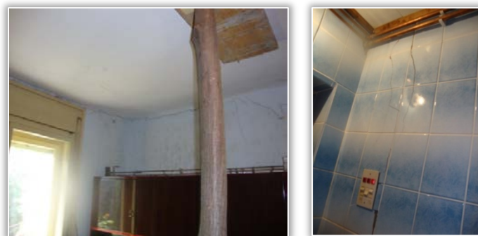
Figure 5. Damage to the ceiling (left) and damage to the ceramic tiles (right)
