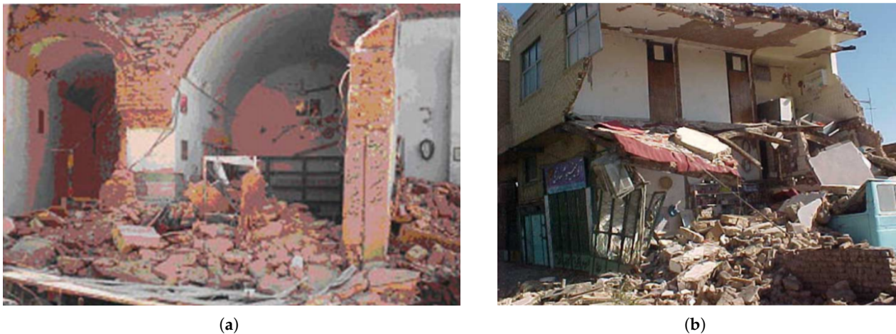
Figure 4. (a) Partially damaged old masonry buildings' arch roofs in Bam after the earthquake [31]; (b) the inconsistency of the multi-arched roof with the supports due to the lack of horizontal coils, as well as the high thickness and weight of the roof [31].
