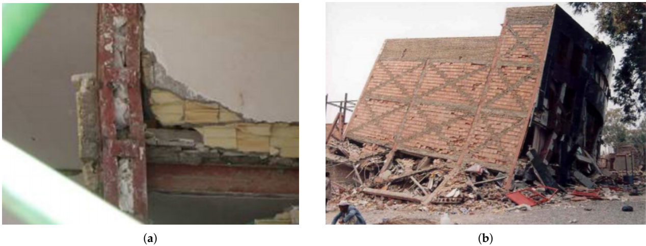
Figure 6. Other types of failures in structural systems [34]; (a) buckling of a column in ground floor connected to the balcony beam; (b) inappropriate lateral bracing system and longer length of first floor column led to a soft story building.
