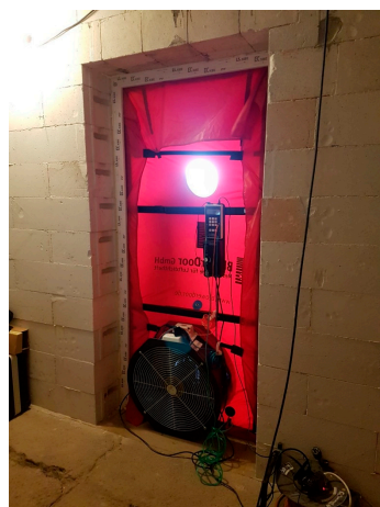
Figure 6. Blower door equipment installed and measurements of test chamber airtightness in progress.
