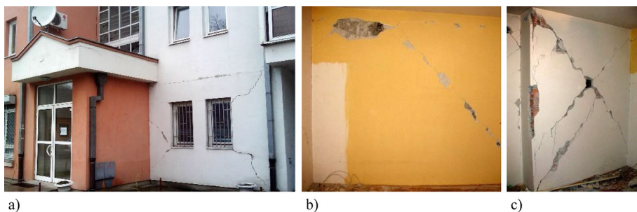
Fig. 30 Performance of type M3-M multi-family residential buildings in the 2010 Kraljevo, Serbia earthquake: a diagonal and horizontal cracks in an exterior wall; b in-plane damage of a load-bearing interior wall (solid clay bricks), and c extensive cracking in a partition wall (multi-perforated clay blocks) (Blagojević 2022)
