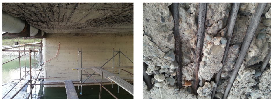
Figure 5. Damage of the superstructure soffit.
