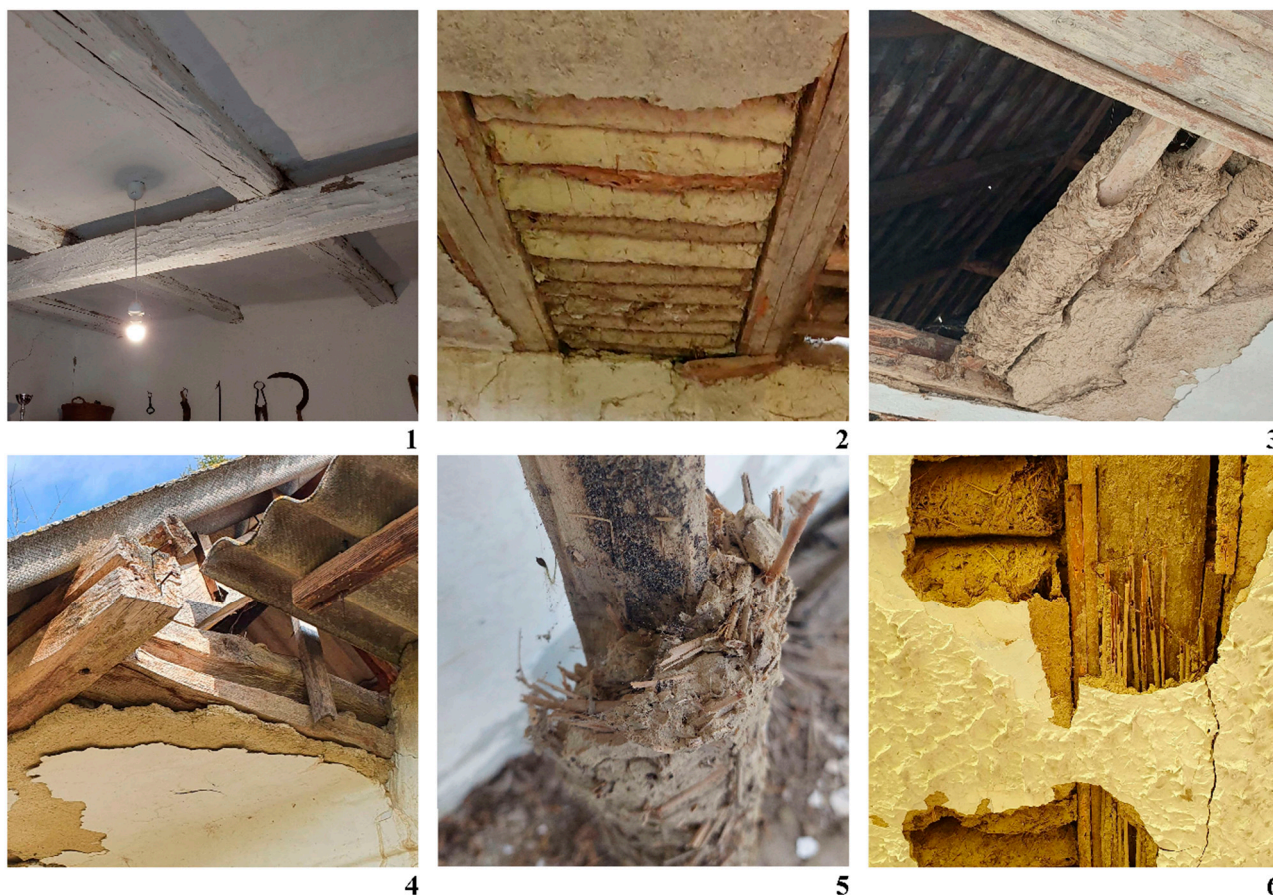
Figure 7. Structural solutions for wooden ceilings in rammed earth houses: (1)—exposed timber beam with joists; (2)—ceiling with vitlovi ; (3)— vitlovi placed between the beams on the battens nailed to the sides; (4)— vitlovi placed in grooves cut into the beams; (5)—detail of vitlovi ; (6)—wooden formwork placed on the underside of the beams. Author’s photos.
