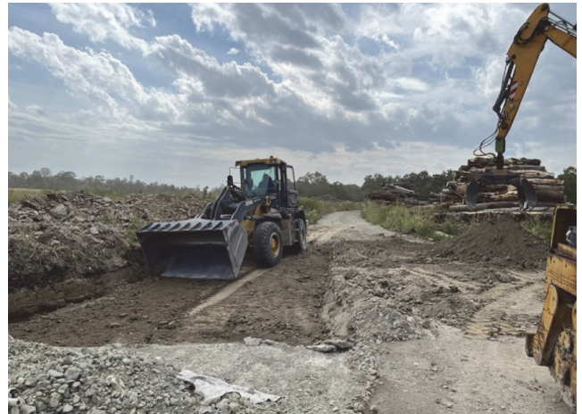
Figure 11. The spreading of the mixture of wood ash and material from the excavation
