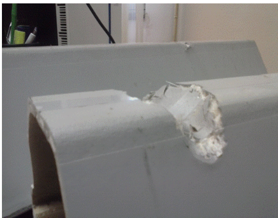
Figure 4. Photograph of beam deformation
