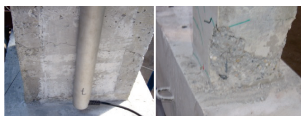
Figure 10 Crack patterns observed on the MODEL 10 columns
