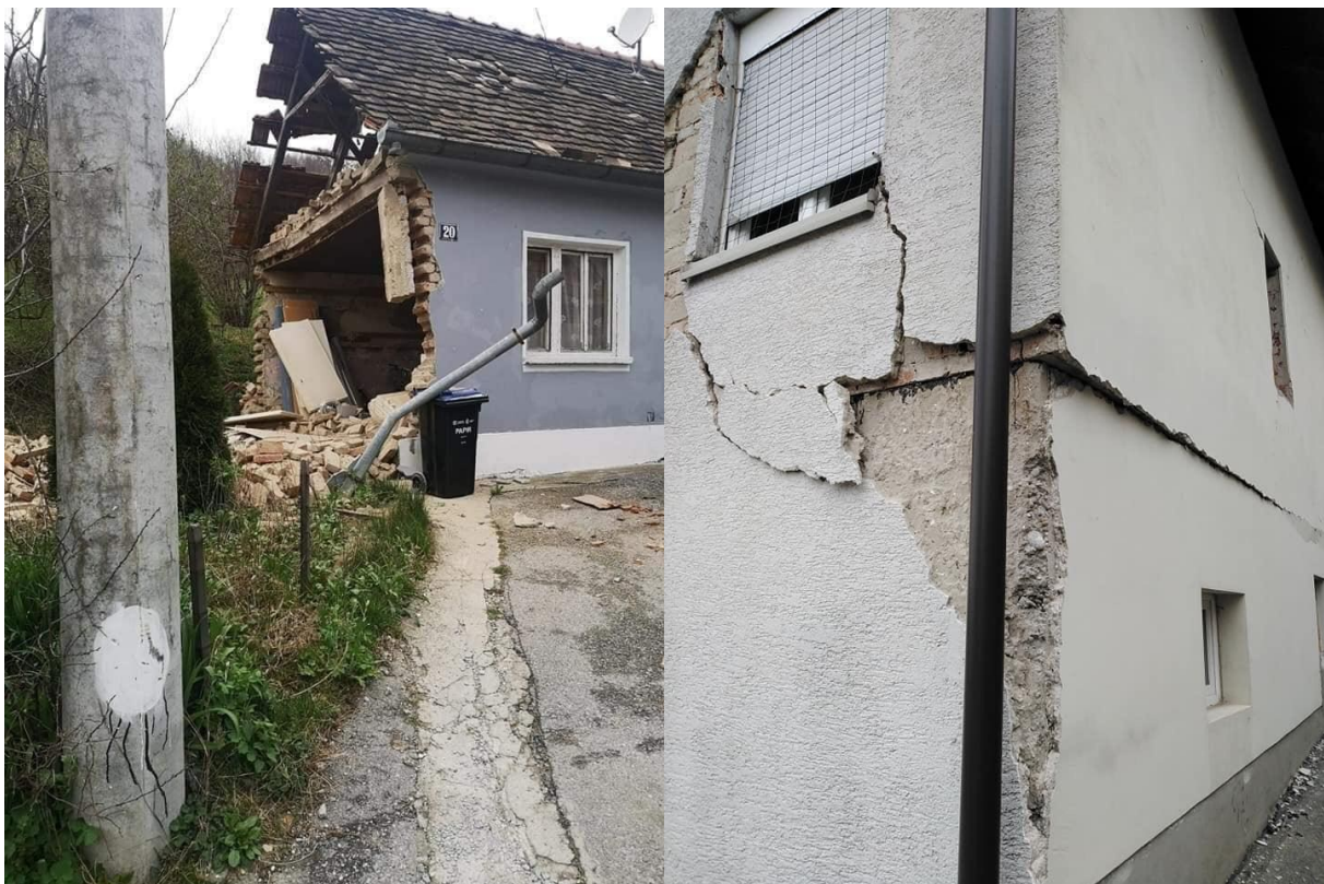
Figure 8. Heavily damaged family house near the epicenter. https://dnevnik.hr/vijesti/hrvatska/potres-u-zagrebu-ostali-bez-domova---598777.html
