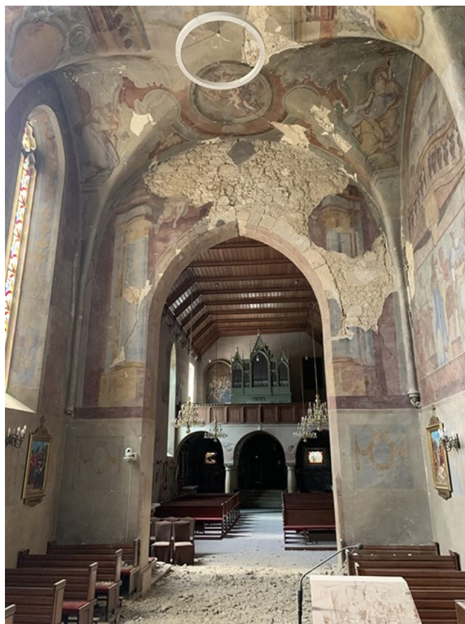
Figure 7. Damage to cultural heritage: Shrine of Saint Mary of Remete from 1786 https://www.24sata.hr/news/pogledajte-trenutak-potresa-u-crkvi-u-remetama-u-zagrebu-682565
