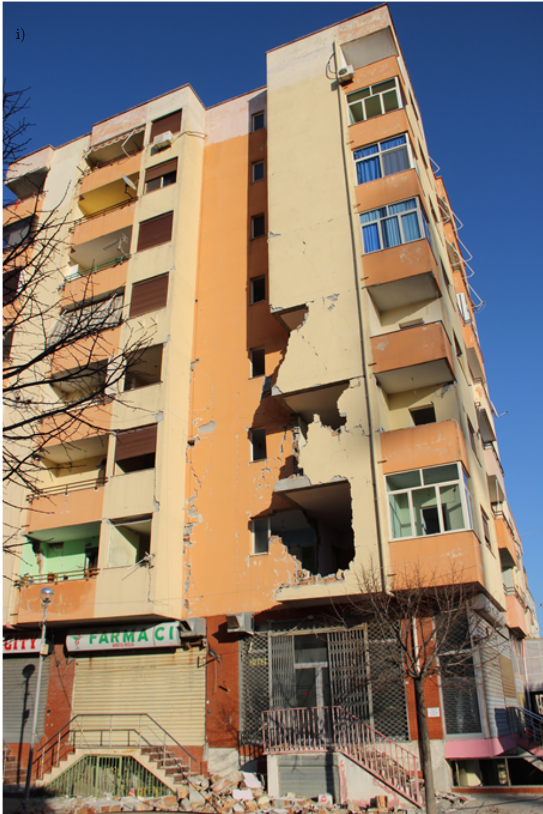
Figure 1.10 (cont.): Damages to the infill walls
