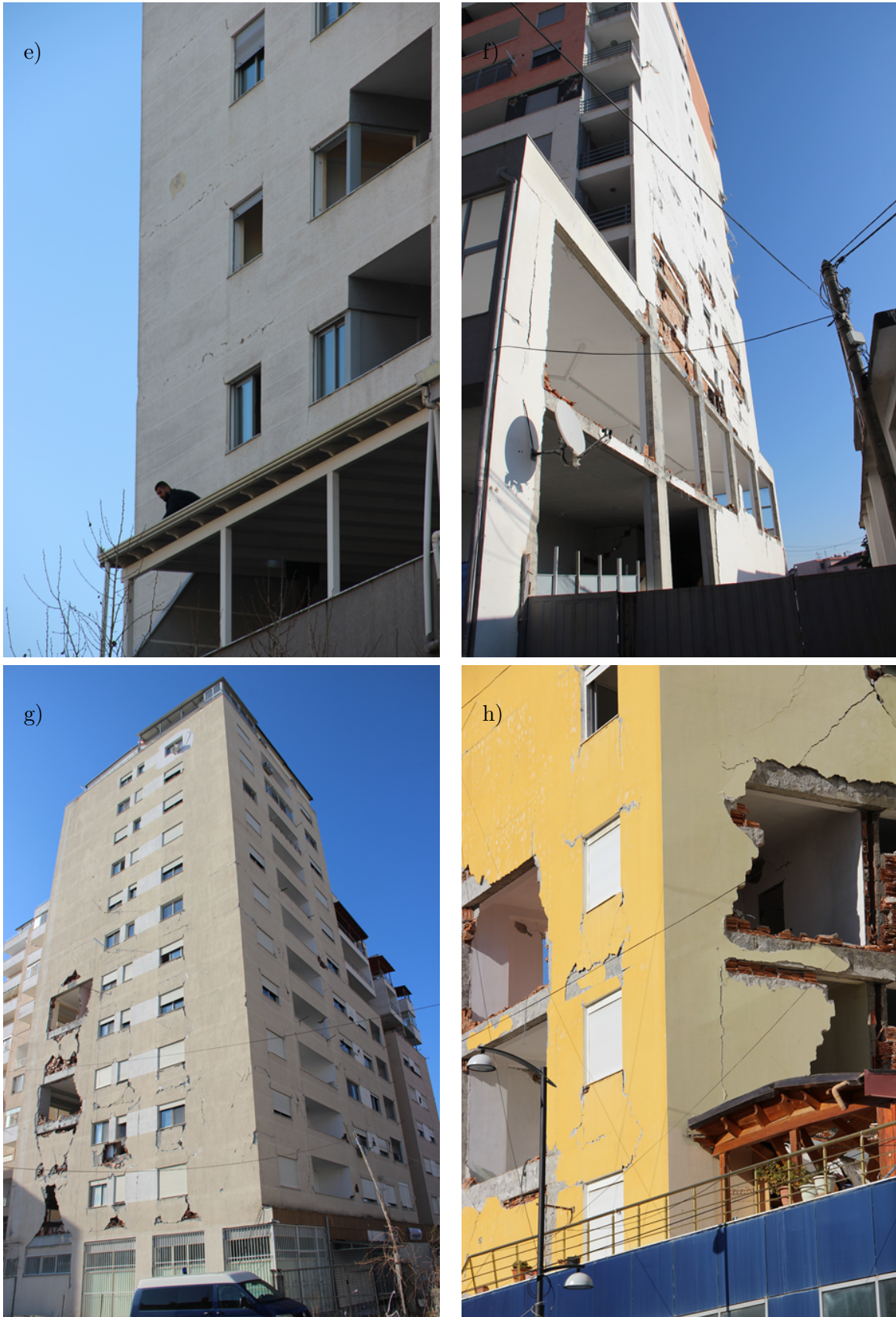
Figure 1.10 (cont.): Damages to the infill walls
