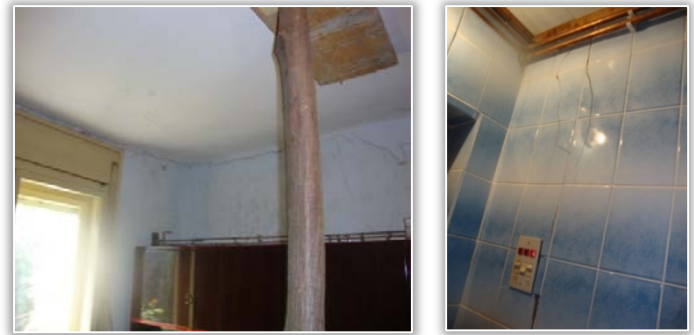
Figure 5. Damage to the ceiling (left) and damage to the ceramic tiles (right)
