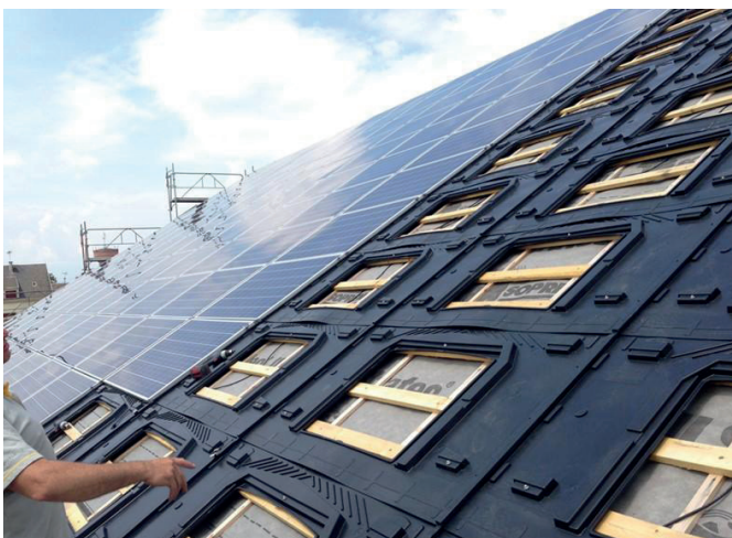
Figure 2. Photovoltaic panels on the roof of a new building, [3]
