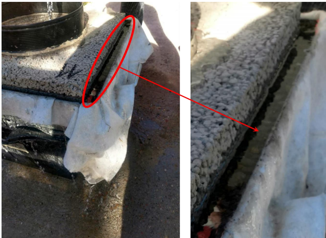
Figure 9. Water film as a result of a discrepancy in pervious concrete infiltration and unbound base course (UBC) exfiltration.
