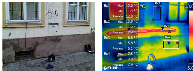
Figure 20. Homogeneous thermal pattern on excitation along the wall.
