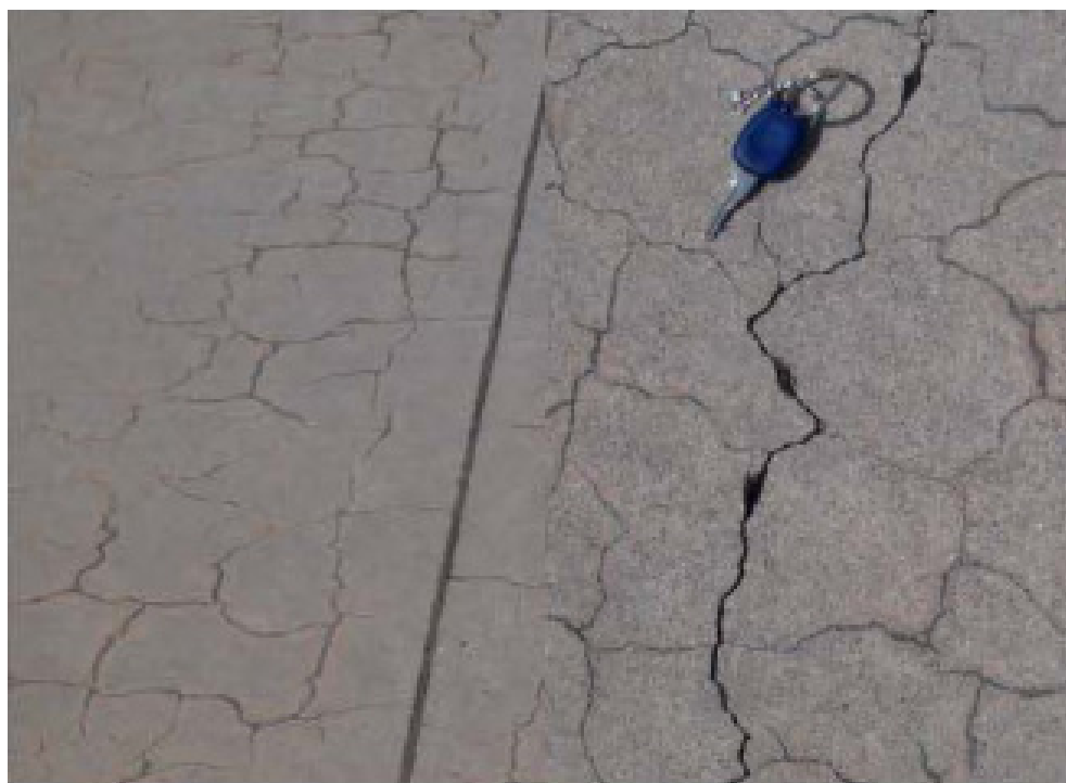
Figure 1. ASR impact on concrete.
