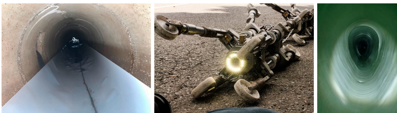
Figure 13. Renewal method—the CIPP method. Adapted with permission from ref. [102]. Copyright 2022 Solmex d.o.o.
