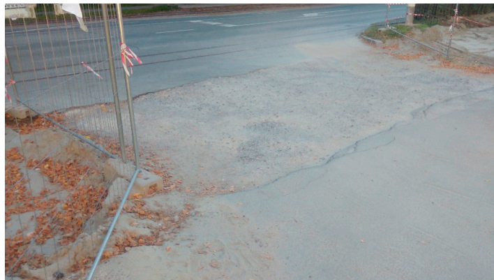
Figure 9. Destroyed asphalt pavement (Photo by D. Obradović).
