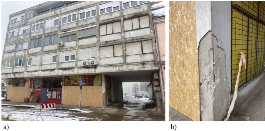
Fig. 33 Damage of type RC1 residential building in Petrinja, Croatia due to the December 2020 earthquake: a exterior view showing open ground floor space which used as a store before the earthquake, and b a detail of the damaged RC column (SUZI-SAE 2021)
