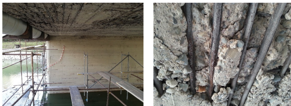
Figure 5. Damage of the superstructure soffit.
