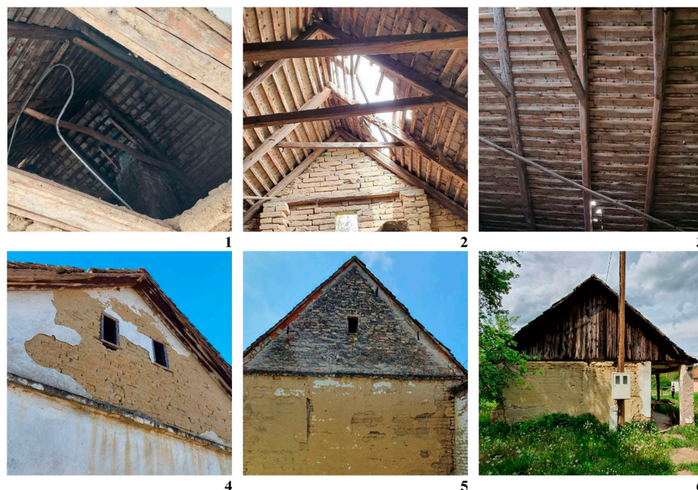
Figure 8. Traditional gabled wooden roofs: (1)—pair of rafters form a triangle with a ceiling joint; (2)—pair of rafters stiffened with a collar tie; (3)—reinforcement with timber wind braces; (4)—adobe gable; (5)—brick gable; (6)—wooden gable. Author’s photos.
