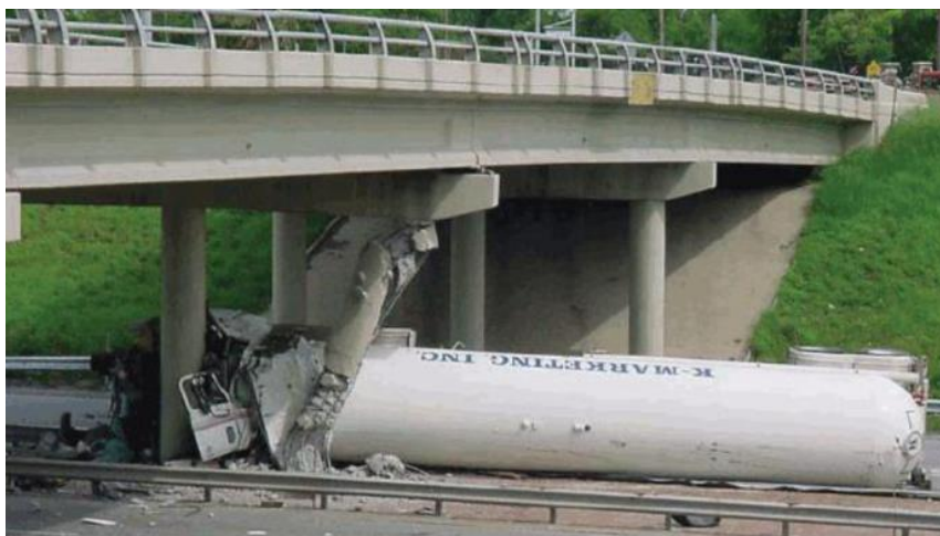
Figure 1 Impact between vehicle and column (U.S. highway) [8]
