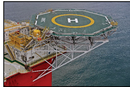
Figure 7 Aluminium helideck on an offshore platform [36]
