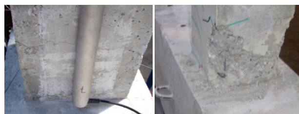
Figure 10 Crack patterns observed on the MODEL 10 columns
