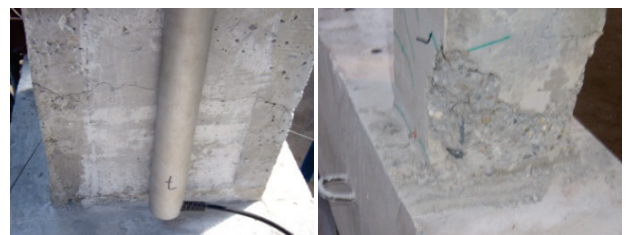
Figure 10 Crack patterns observed on the MODEL 10 columns
