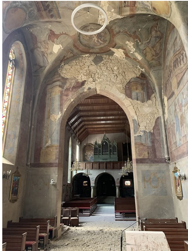
Figure 7. Damage to cultural heritage: Shrine of Saint Mary of Remete from 1786 https://www.24sata.hr/news/pogledajte-trenutak-potresa-u-crkvi-u-remetama-u-zagrebu-682565
