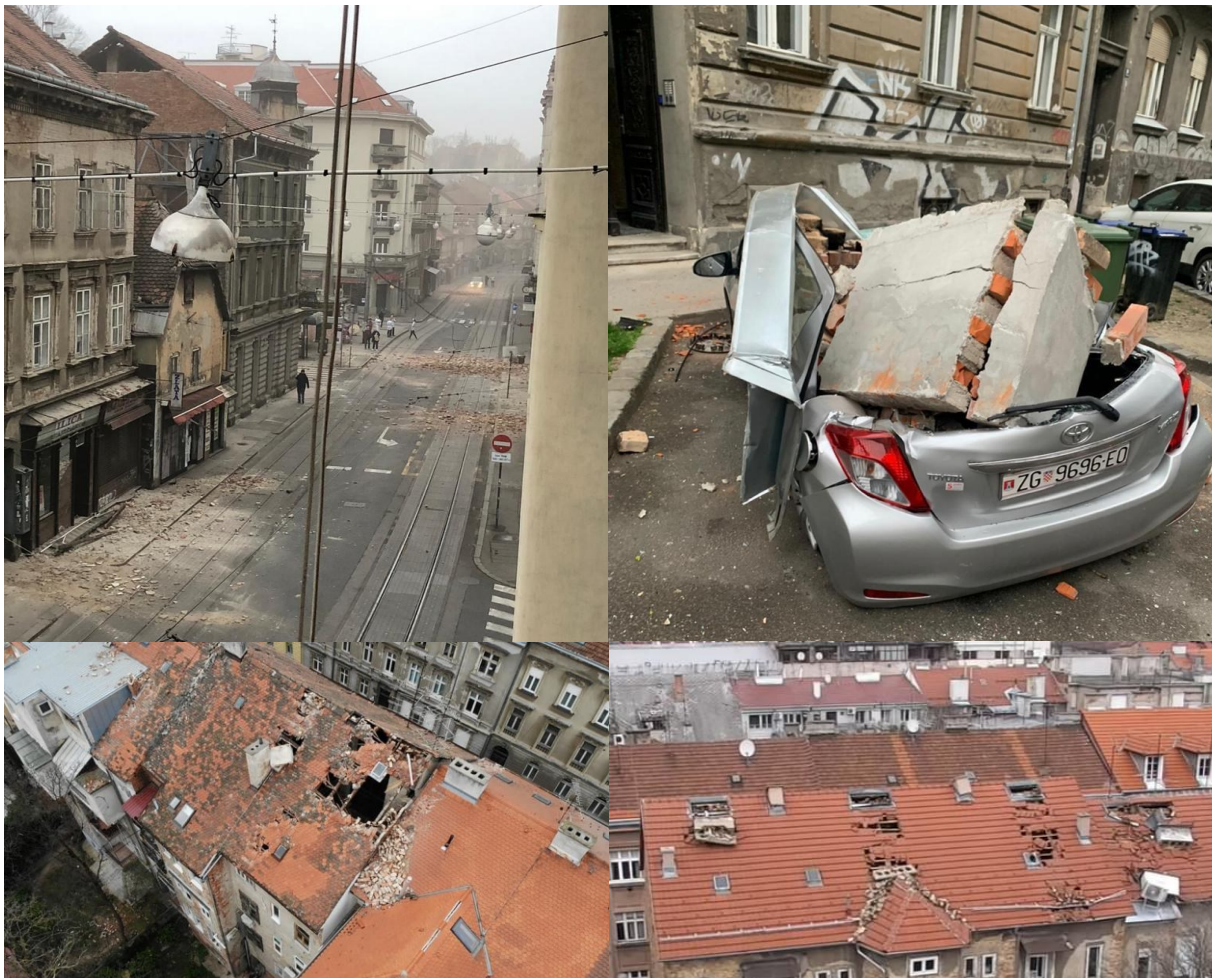
Figure 5. Damage in Zagreb after 22 March M5.5 earthquake. Noticeable roof tile loss and chimney collapse
