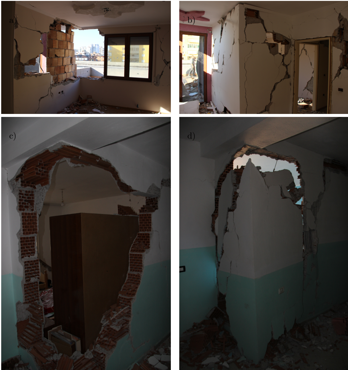
Figure 1.10: Damages to the infill walls
