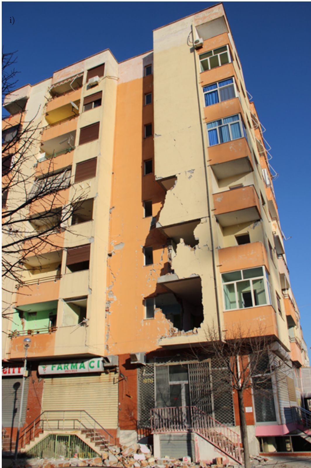
Figure 1.10 (cont.): Damages to the infill walls
