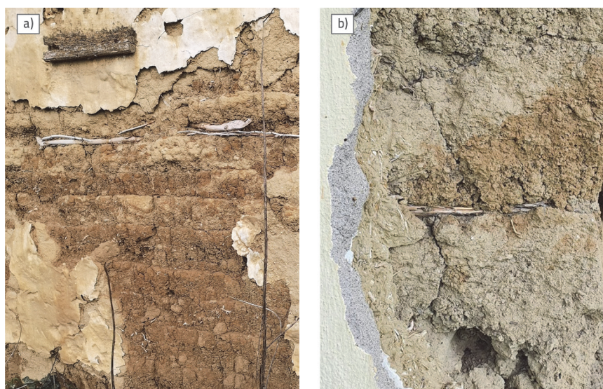
Figure 7. Rammed-earth walls from eastern Croatia with organic material between compacted layers (author's photos): a) brushwood, b) reed and chaff
