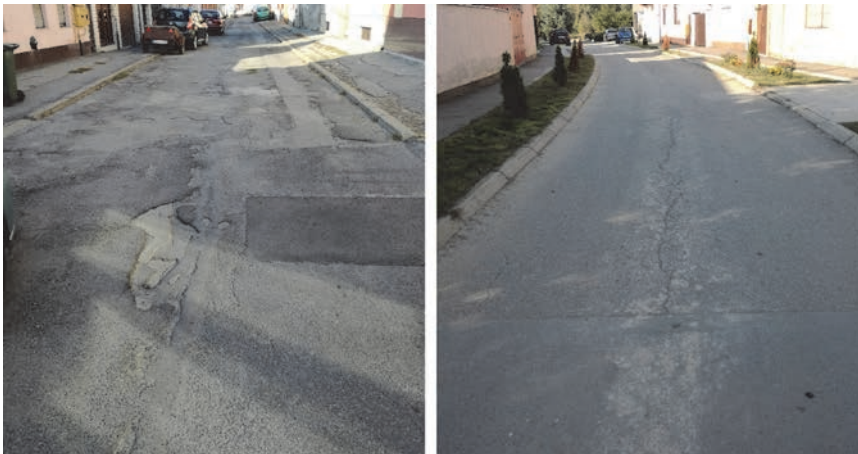
Figure 7. Photographs of actual pavement condition: a) Cvjetkova Street, b) Lađarska Street
