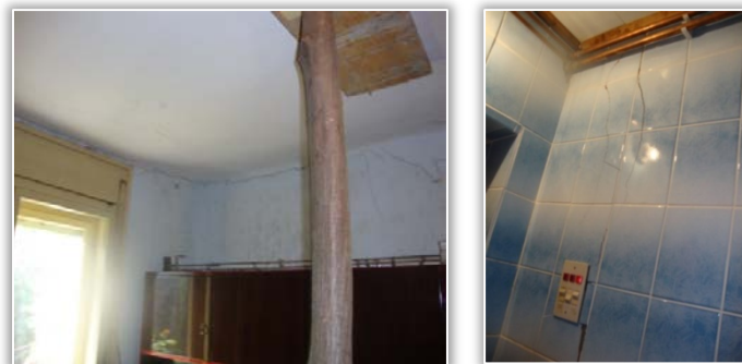
Figure 5. Damage to the ceiling (left) and damage to the ceramic tiles (right)
