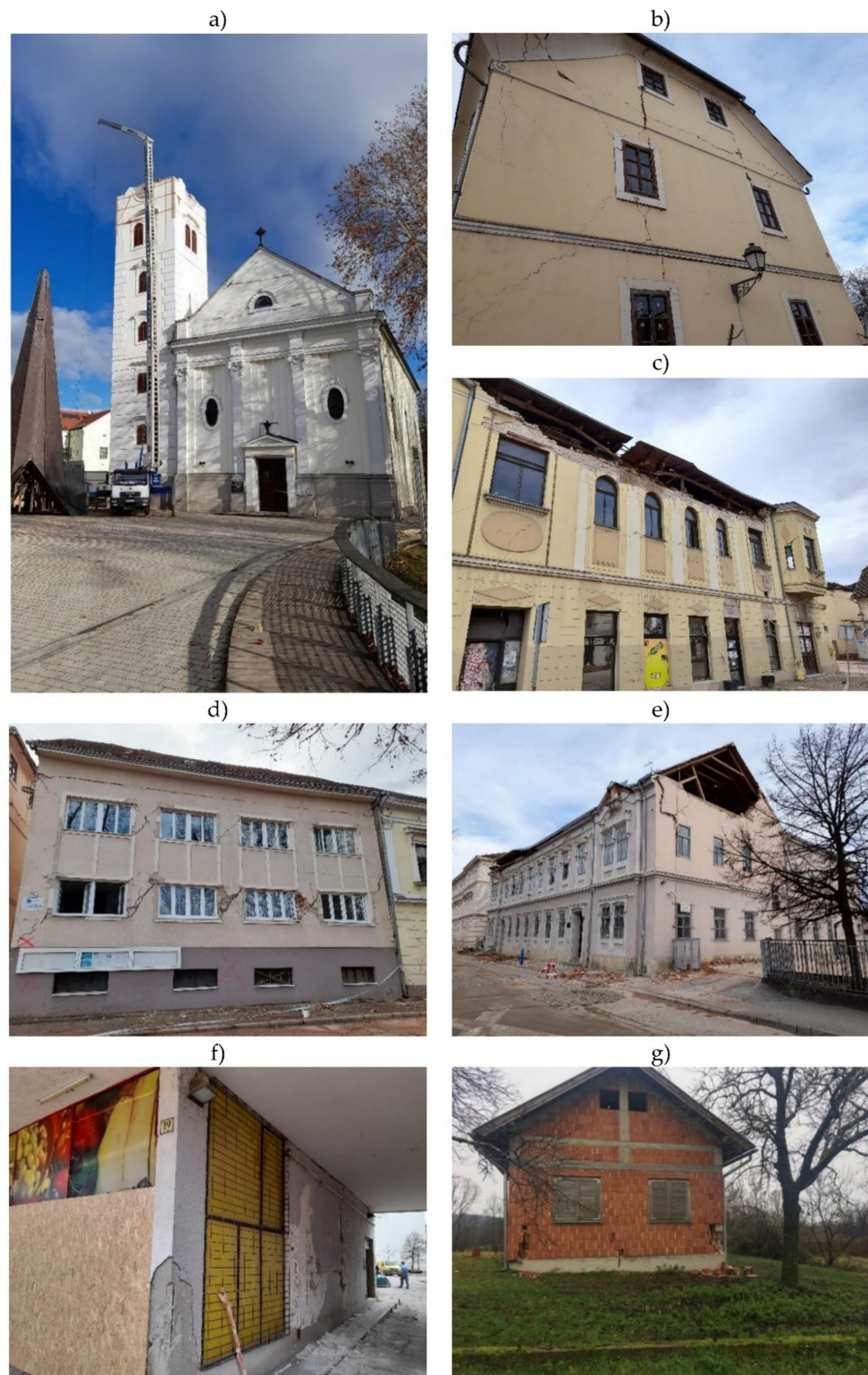
Figure 11. Damages that were sustained by various building types built in the pre-code era (before 1964) and in various code eras: (a) The Cathedral of the Exaltation of the Holy Cross in Sisak with the tower roof removed; (b) Crack distribution in an old masonry building in Petrinja; (c) Parapet wall collapse in an old masonry building in Petrinja; (d) Masonry pier diagonal tension cracking; (e) Gable wall out-of-plane collapse in an elementary school in Petrinja; (f) Damage to the masonry-infilled RC frame (soft storey collapse); and (g) Damage to a building that was built without vertical confining elements as part of a rebuilding programme in the post-war era [58] (author of all photos: D. Penava).
