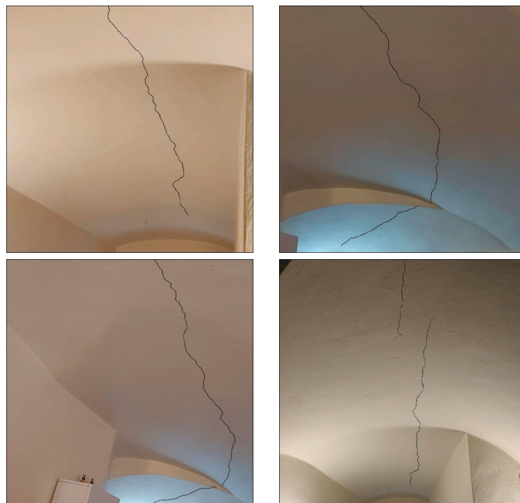
Figure 13. Damage observed on ceiling vault of the west tower at ground floor (damage ID on all four images is 13 in Figure 10a).
