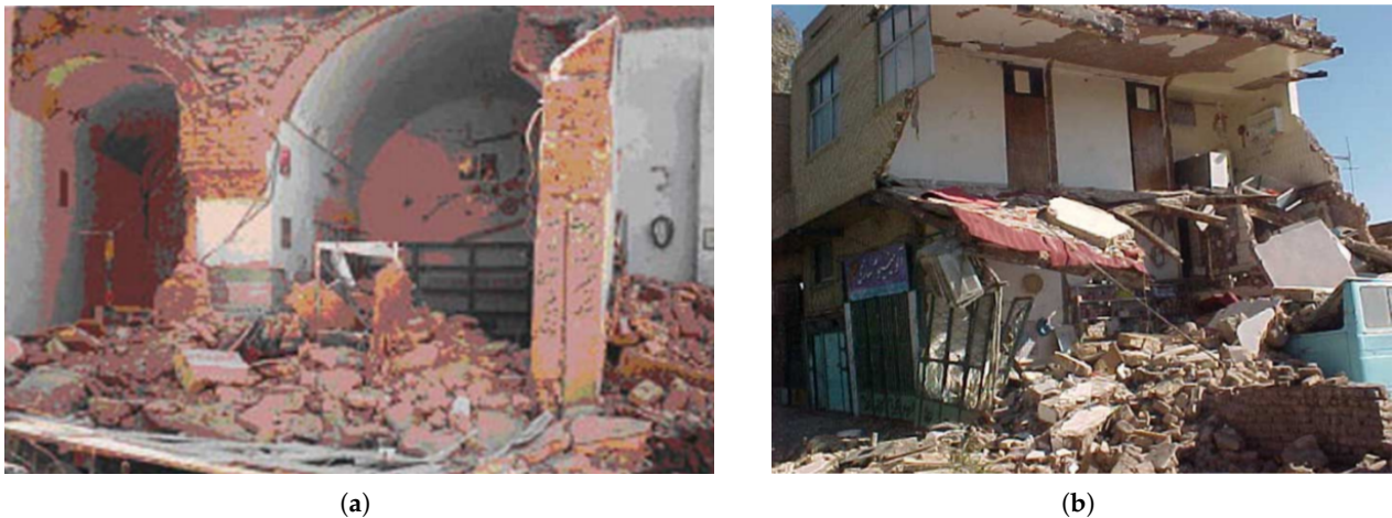
Figure 4. (a) Partially damaged old masonry buildings' arch roofs in Bam after the earthquake [31]; (b) the inconsistency of the multi-arched roof with the supports due to the lack of horizontal coils, as well as the high thickness and weight of the roof [31].
