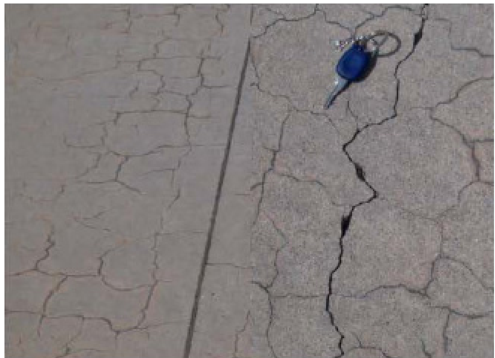
Figure 1. ASR impact on concrete.
