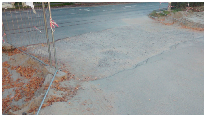
Figure 9. Destroyed asphalt pavement (Photo by D. Obradović).
