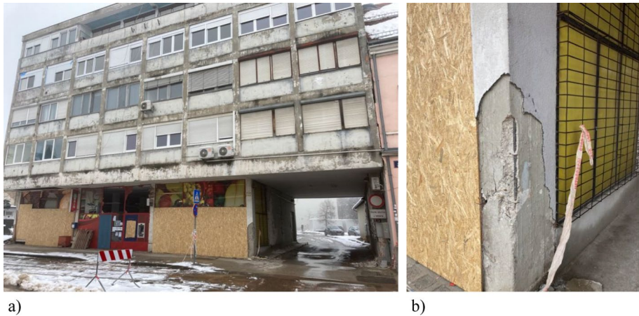
Fig. 33 Damage of type RC1 residential building in Petrinja, Croatia due to the December 2020 earthquake: a exterior view showing open ground floor space which used as a store before the earthquake, and b a detail of the damaged RC column (SUZI-SAAE 2021)
