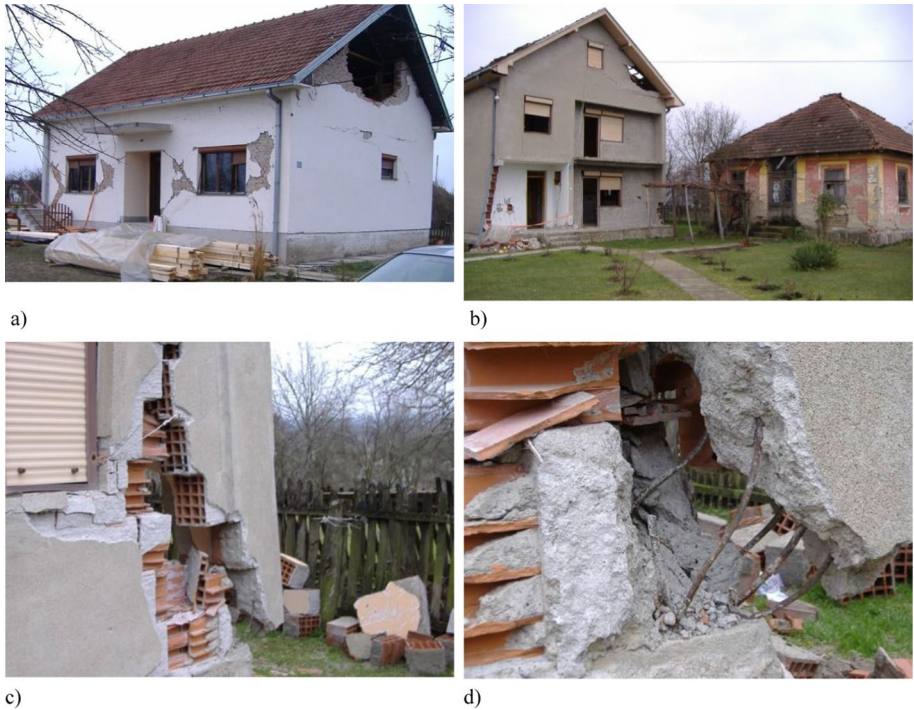
Fig. 28 Rural single-family masonry buildings affected by the 2010 Kraljevo, Serbia earthquake: a a severely damaged type M2 building; b a damaged inadequately confined M4 type building (left) adjacent to an undamaged old timber-frame (bondruk) building; c and d damage at the corners of the building shown in figure b due to construction flaws (Manić and Bulajić 2014)
