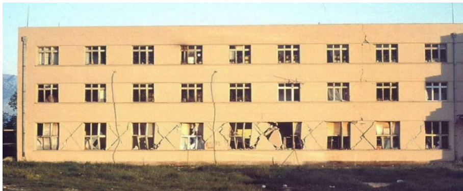
Fig. 25 Budva Town Hall—an example of a type M3-M building damaged in the 1979 Montenegro earthquake (M. Fischinger)
