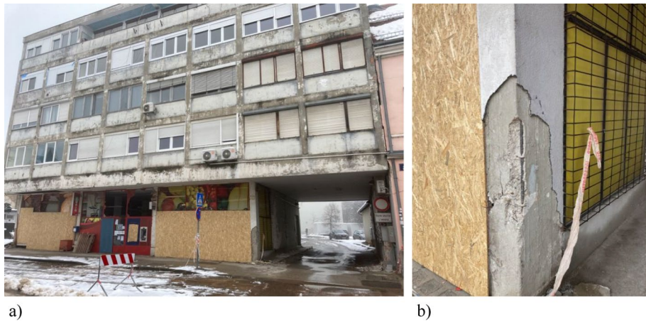
Fig. 33 Damage of type RC1 residential building in Petrinja, Croatia due to the December 2020 earthquake: a exterior view showing open ground floor space which used as a store before the earthquake, and b a detail of the damaged RC column (SUZI-SAE 2021)
