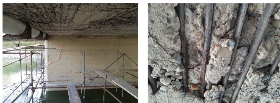
Figure 5. Damage of the superstructure soffit.
