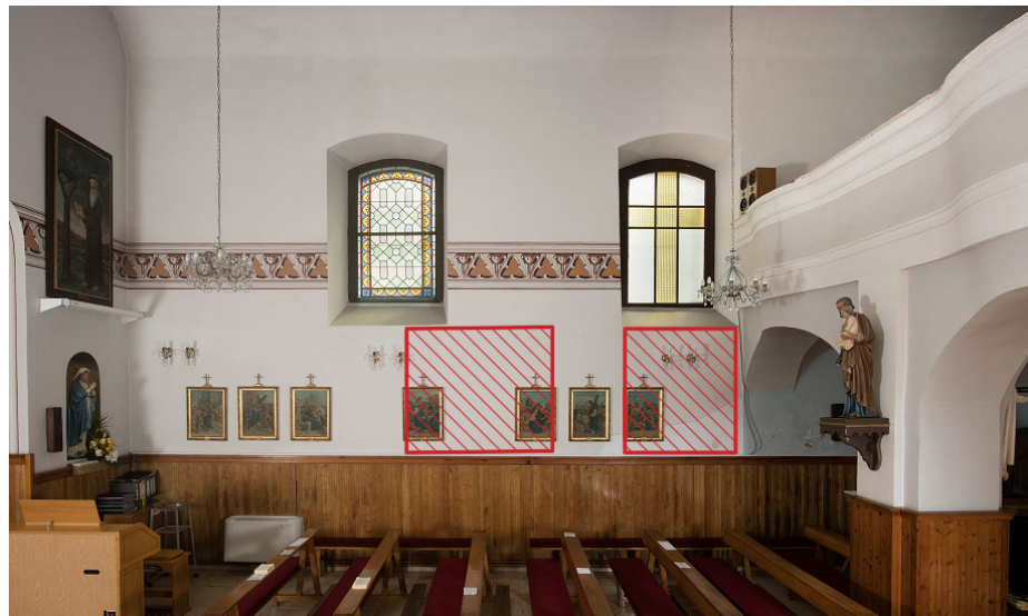
Figure 12. Southern wall with marked area made of different material.
