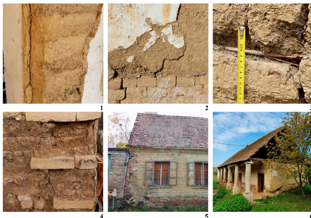
Figure 6. Construction details of rammed earth walls: (1)—RE layers (app. 10 cm); (2)—RE wall built on a layer of planks on a brick base; (3)—RE layers reinforcements; (4)—corner reinforced with layers of reeds or wickerwork; (5): brick corners and columns set into the wall; (6)—columns with a round cross-section. Author’s photos.
