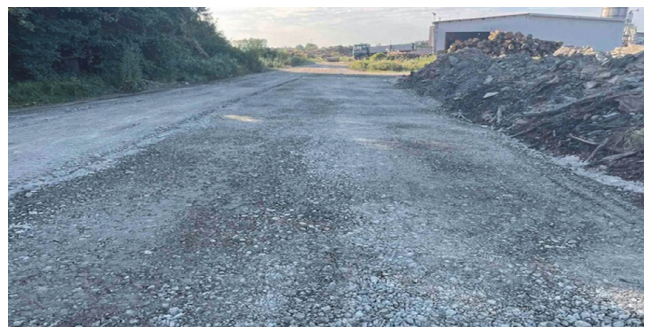
Figure 8. The constructed unbound pavement of the internal road made of crushed stone [32]
