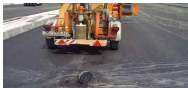
Figure 7. Sample taken at the Odra Viaduct from the completed waterproofing – asphalt system
